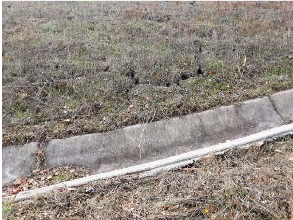
Photo 19. Soil cracks and creep impacting v-ditch behind 25 Maplewood Drive.
