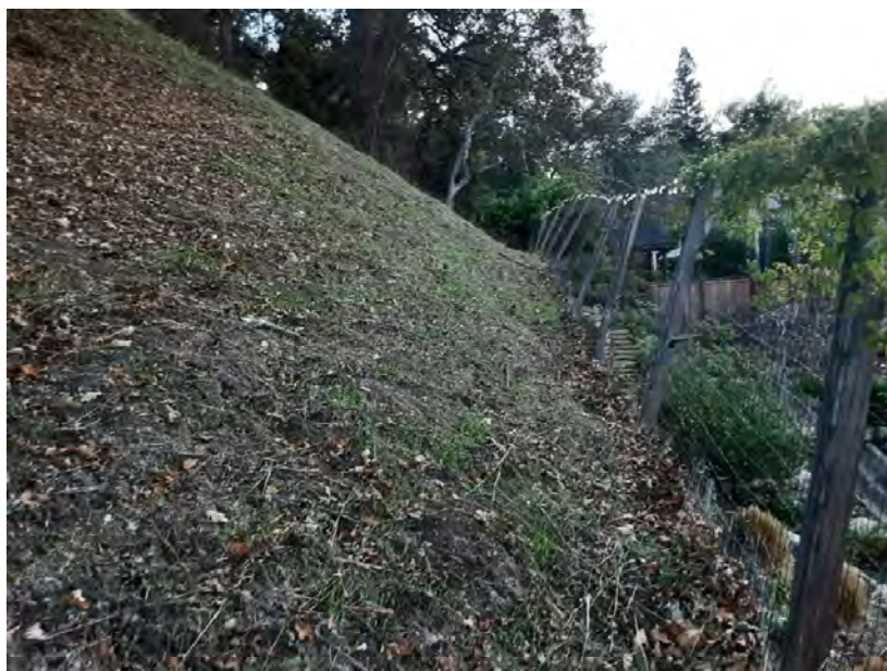
Photo 6. View of creep impacting the fence behind 120 Windover Drive.
