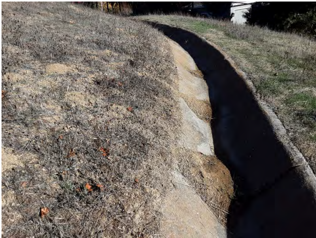
Photo 8. View of burrow holes depositing sediment into v-ditch behind 7 Crownridge Drive.
