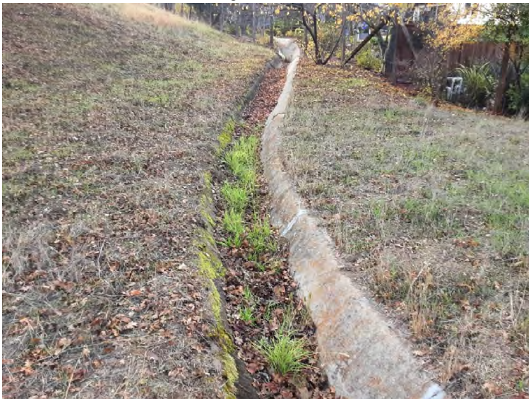
Photo 22. Significant amount of debris and grass growing in v-ditch behind 116 Leaffield Rd.
