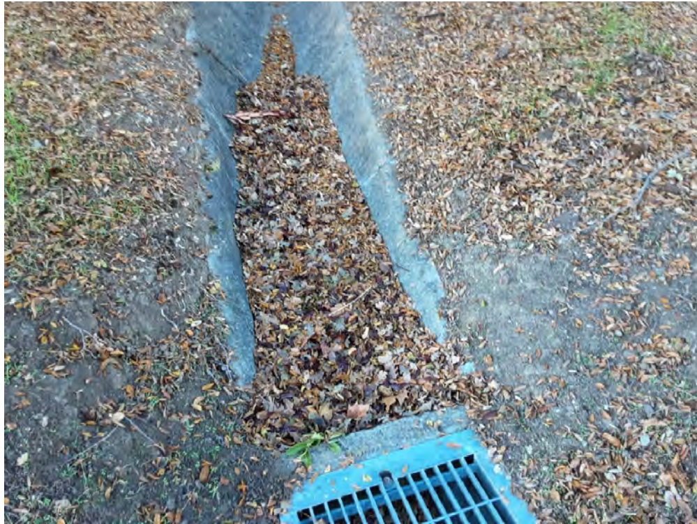
Photo 21. Debris blocking direct inlet at 154 Sunhaven Road.
