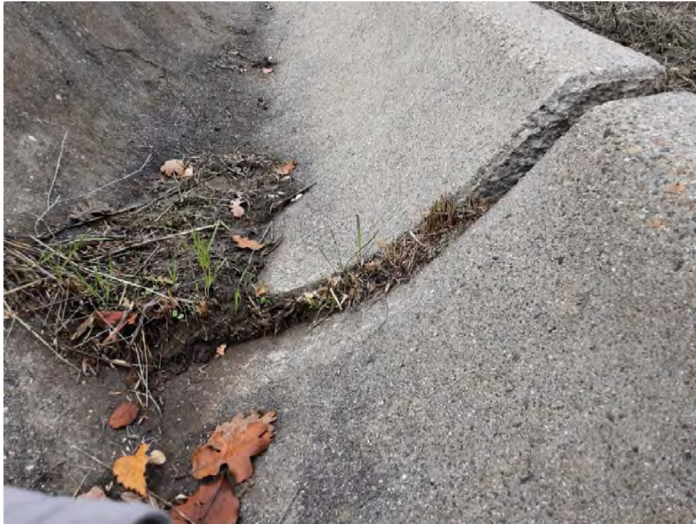
Photo 17. Vertical offset of 1.5 inches at v-ditch behind 25 Maplewood Drive.
