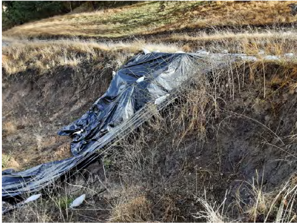
Photo 11. Slope failure on the eastern bank of the fire road south of 138 Windover Drive.
