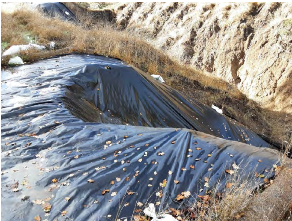
Photo 12. Slope failure on the eastern bank of the fire road south of 138 Windover Drive.
