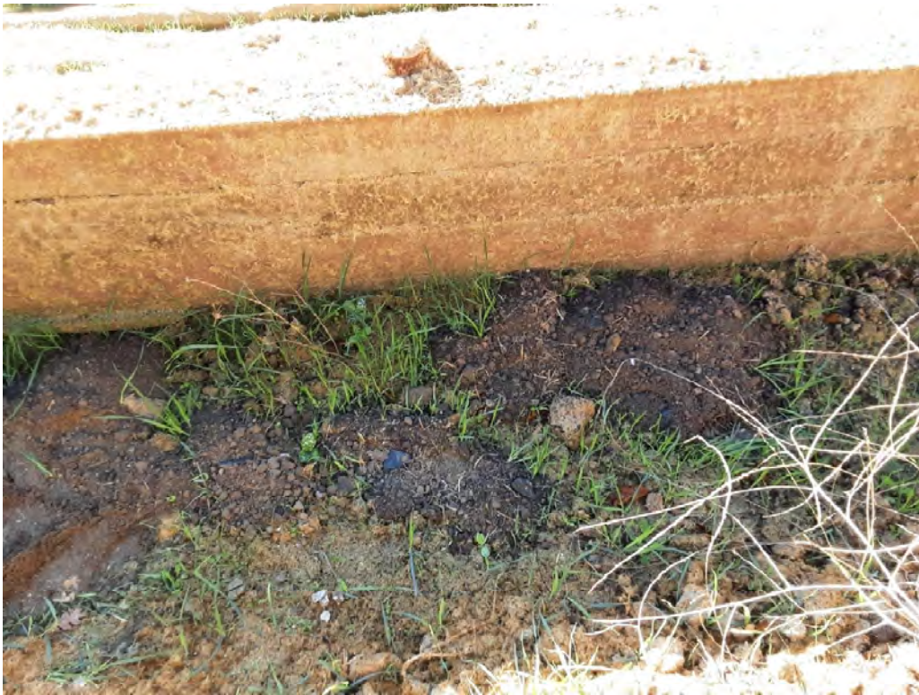
Photo 9. Burrow holes observed at the base of the wood wall built as part of the repair behind 155 & 158 Sunhaven Road.
