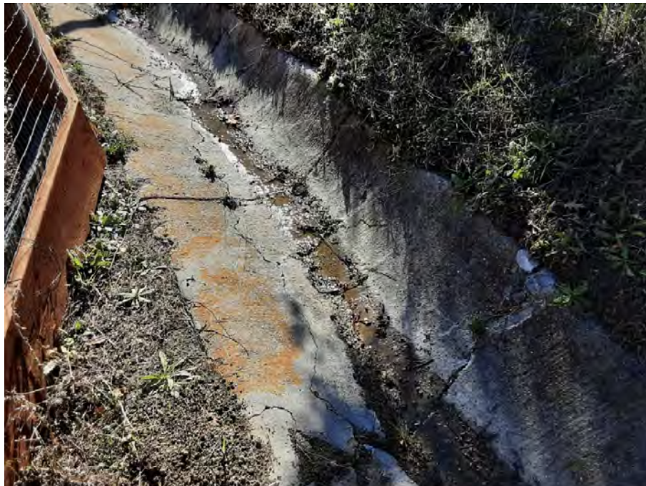
Photo 2. View of v-ditch with cracks and discharge from subdrain pipe.
