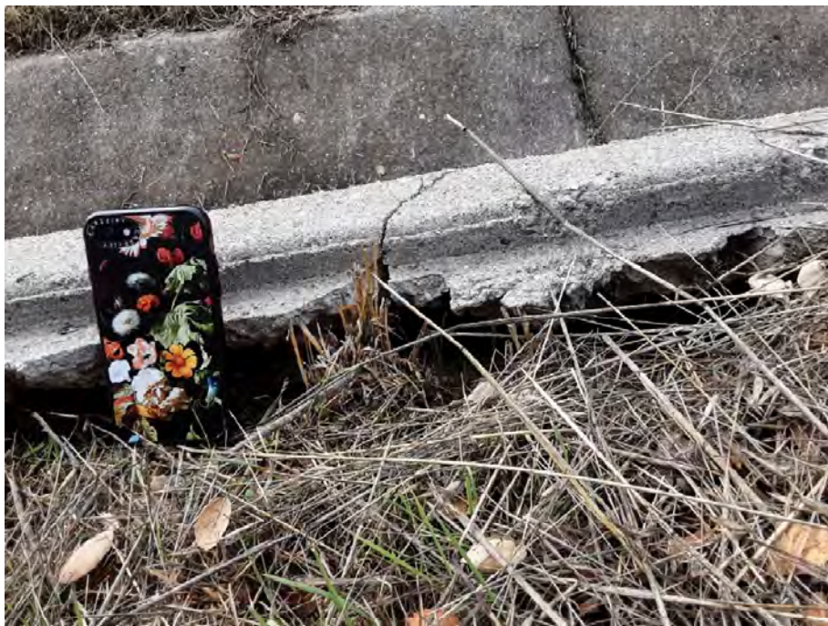
Photo 18. V-ditch lifted 2.5 to 3 inches and cracking from creep behind 25 Maplewood Drive.
