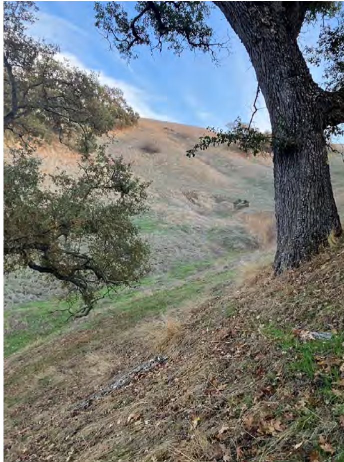
Photo 5. View of recently active landslide in drainage area east of Windover Drive near gabion wall.
