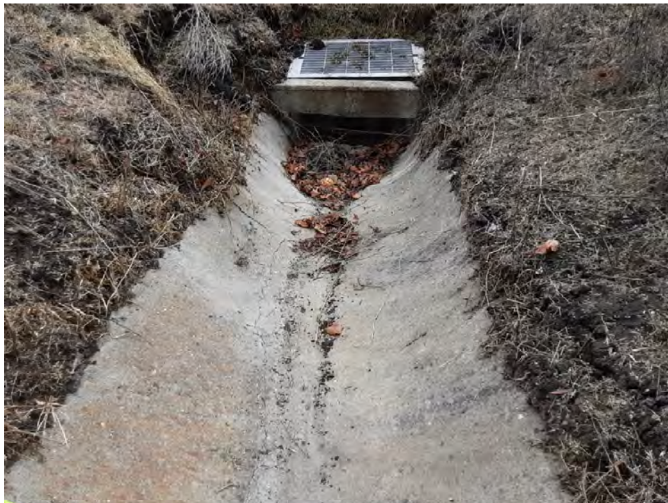
Photo 20. V-ditch and direct inlet behind 19 Maplewood Dr affected by creep, erosion, and debris deposition.
