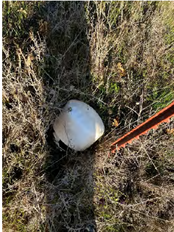
Photo 3. View of a damaged subdrain cleanout riser.
